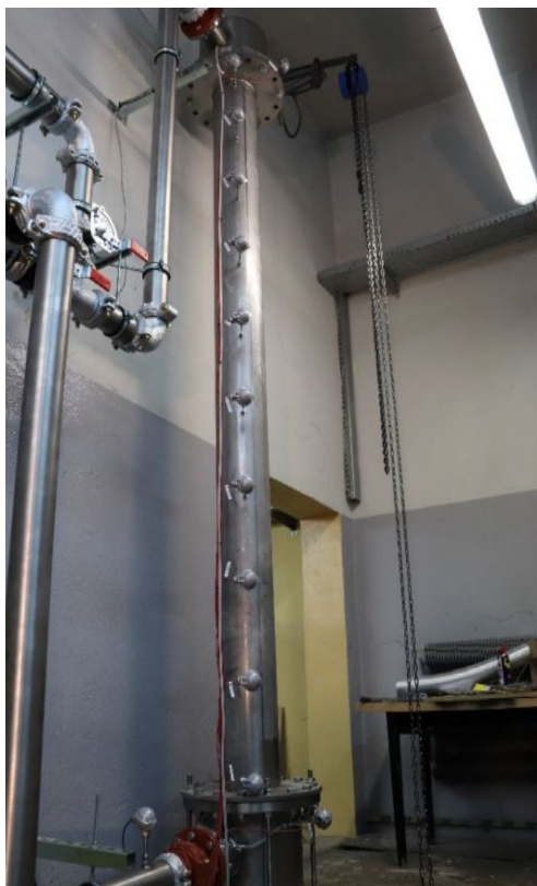
Figure 7: Thermal energy storage tank in a variant without thermal insulation
